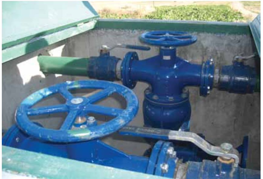
On the valves, there are four solenoids, which receive signal from a SCADA system
