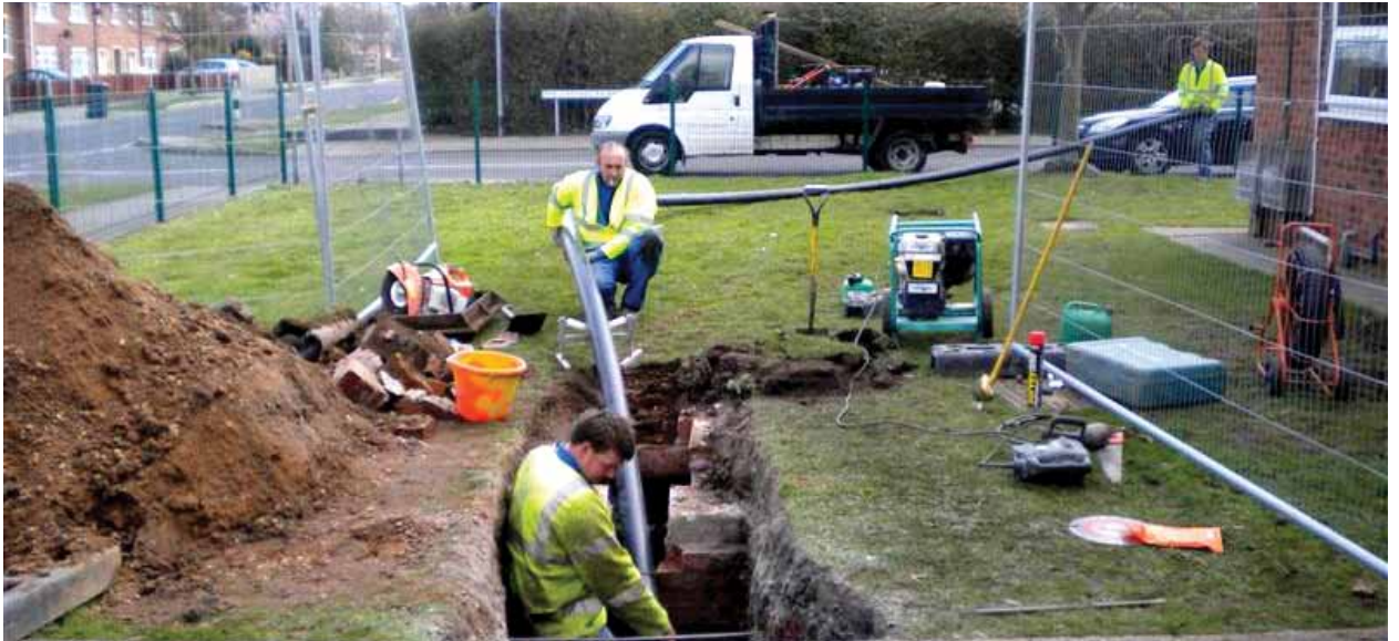
The new pipe being fed into the ground during a bursting run
